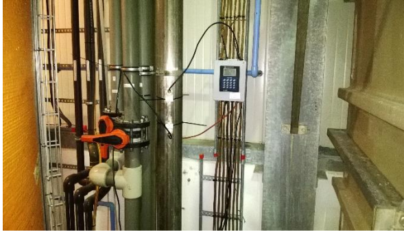
FIGURE 4 Flow measurement of Preox with a portable full pipe flow meter.
